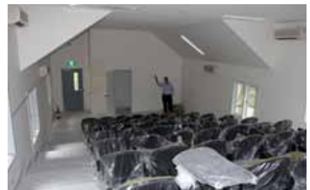
Expanded lecture theatre - almost finished. This updated facility now accommodates more than 70 people. All of the seating has been replaced and air conditioning has been installed.
