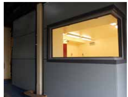
Work-in progress in the aquarium. This room will become the new protected (PC2) laboratory within the SIMS aquarium - one of only two such aquarium facilities in Australia.
