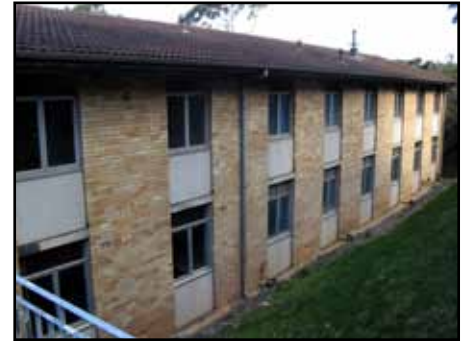
ABOVE: The old barracks Building 19, as seen from the road before renovation.
